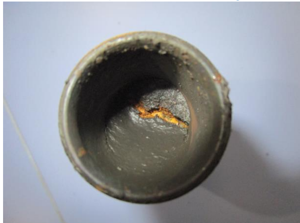
ESFR K25 (2002) dirt at sealing
